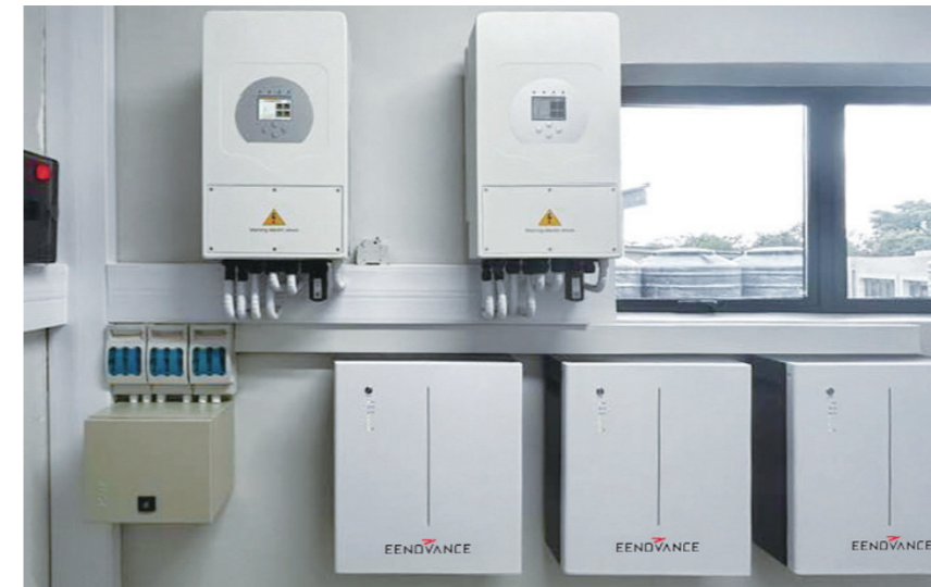
15.96kWh ● August, 2025 ● Location: Germany ■ Configuration: 3 * MANA 5.3 batteries
