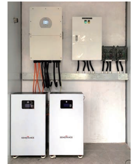
32.14kWh ● July, 2025 ● Location: Pakistan ■ Configuration: 2 * MANA 16.0 batteries
