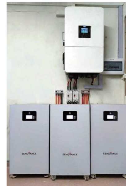
48.21kWh ● December, 2025 ● Location: Philippines ■ Configuration: 3 * MANA 16.0 battery
